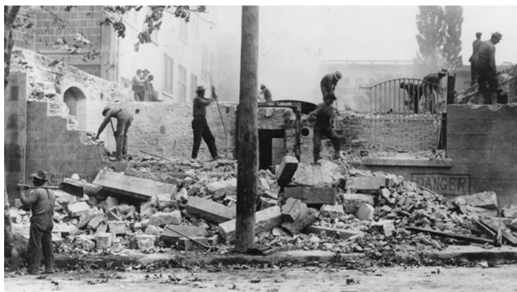
Turn of the century style “shovel ready” courthouse project for Multnomah County. Demolition of the previous courthouse underway.
